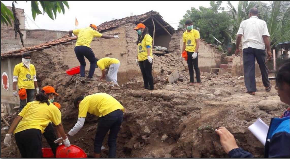
The NSS volunteers have extended their support to the flood-affected villages in Sangli by aiding in the reconstruction of damaged homes
