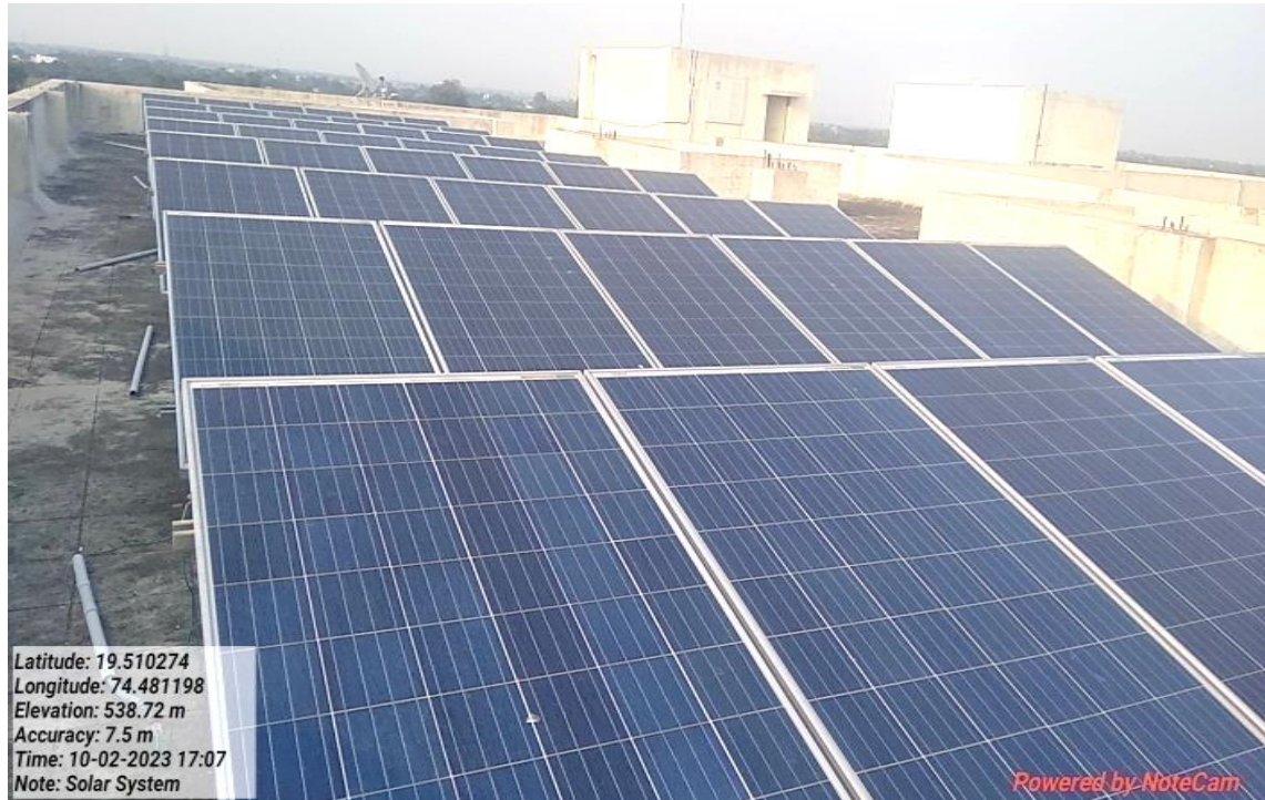
Solar PV System Date:10/02/2023
